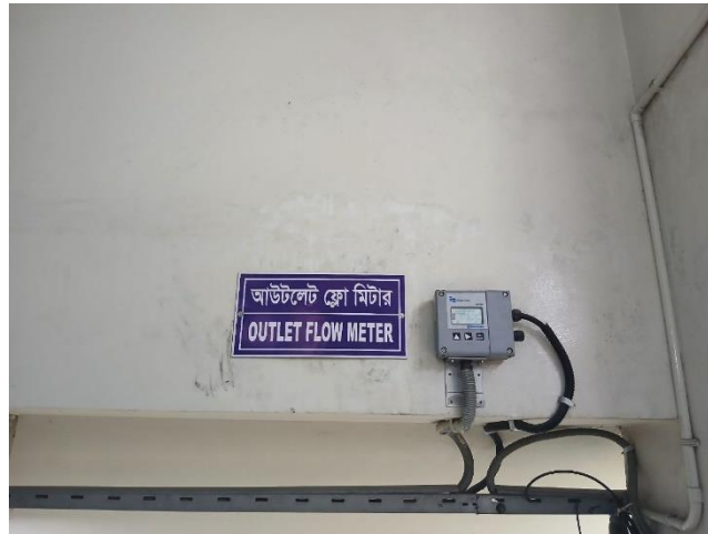
ETP Outlet Flow Meter
