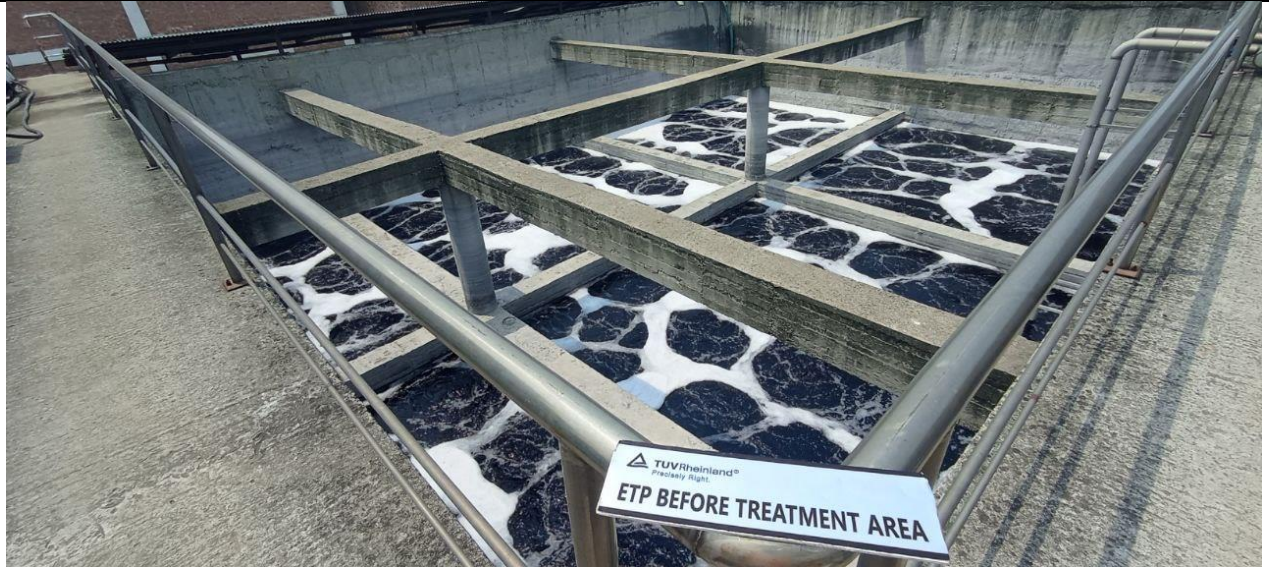
M001- Untreated Wastewater
